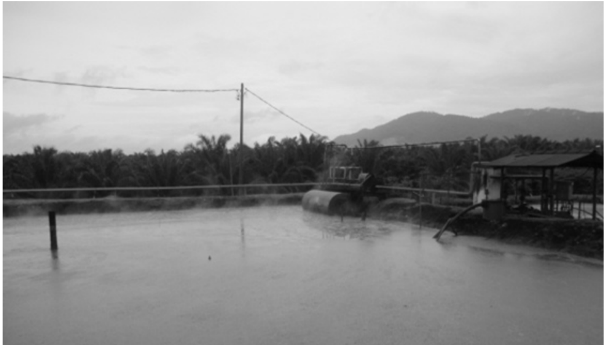
Figure 3: Pump Extracting SPO from Pond
