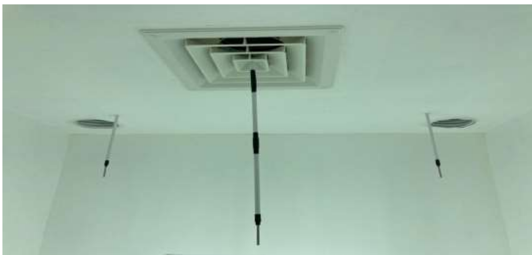
Fig. 1. The installation of square diffuser and thermocouple type-K in chamber
