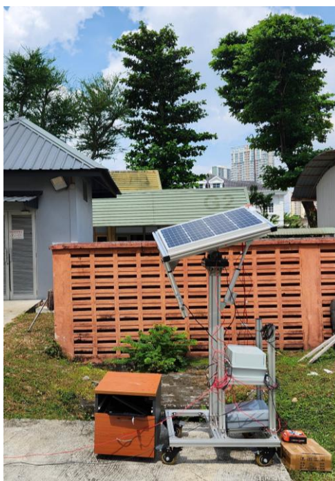
Fig. 5. Solar tracker position outside G3 building UTM
