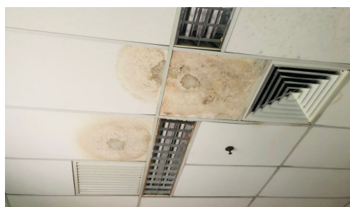
Fig. 2. Watermarks on ceiling due to water drop (condensation)
