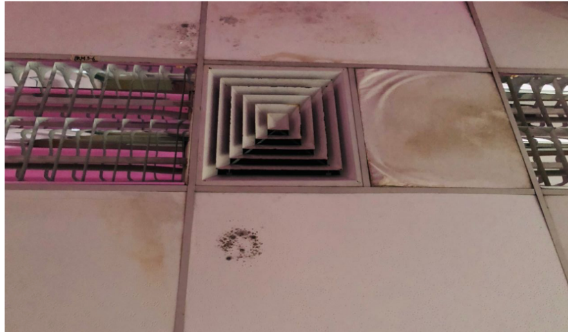
Fig. 3. Ceiling dampness and mould growth
