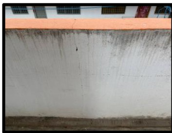
Fig. 1. Crack on balcony wall
