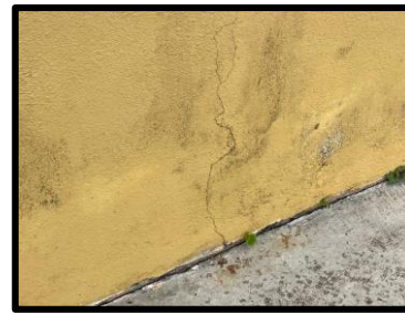
Fig. 4. Crack on the wall
