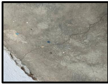
Fig. 3. Crack on the floor
