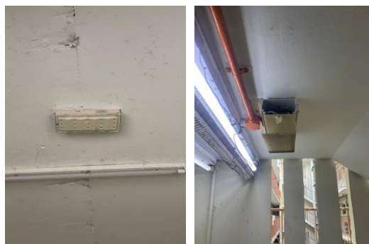
Fig. 6. Emergency lighting system problem
