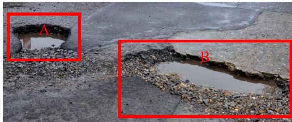
Fig. 3. Pothole with high light exposure
