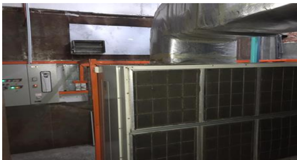
Fig. 1. (b) The air handling unit
